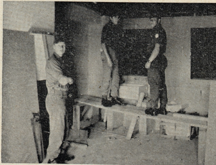
● Sapper "Ginge" Woolnough, Sapper John Boland and Lance Corporal John Sawm at work in the new Sergeants' Mess accommodation.
